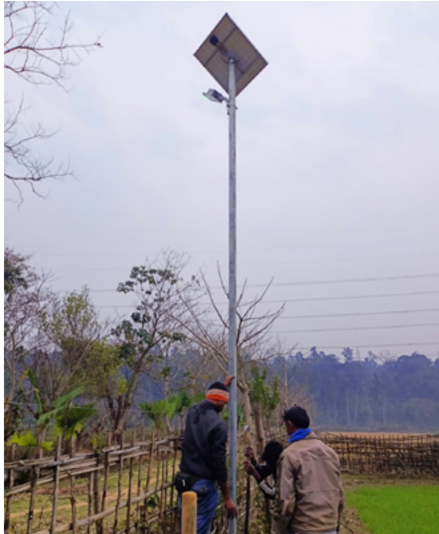
Solar street light system installed in an HEC affected area
